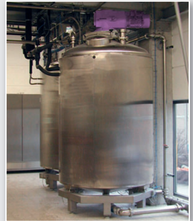
Wheat predough tank with 2 tanks with 4500l capacity each
